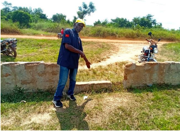
Zwedru UMS PTA chairperson, Mr. Bewehyee, at school fence under construction. Dec. 6, 2023.
