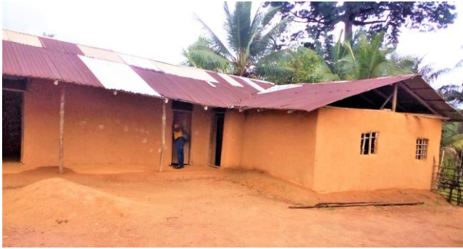
Thomas H. Brewer UMS in Bewahn, Grand Kru County, Garraway District has 38 students in first through fifth grade in this stick and mud building and 48 students in the nursery and kindergarten classes in the church building, September 29, 2022.
