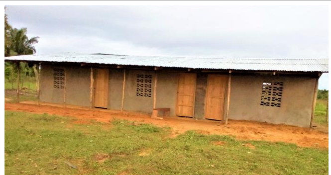
At Anna E. Hall UMS, Garraway Beach, Grand Kru County, Garraway District, the annex work continues. Doors and colombo windows were added. Now chairs are needed so the students can move in. September 28, 2022
