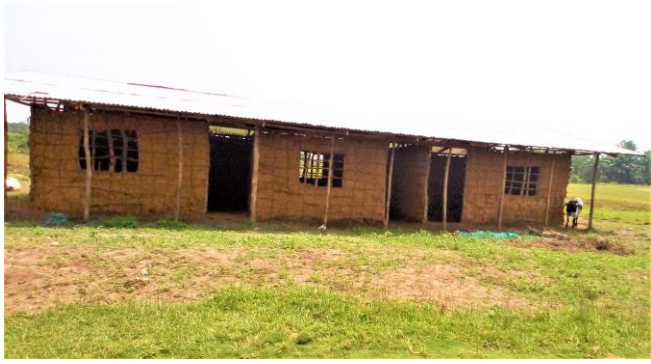
3-classroom annex under construction at the Anna E. Hall Elementary & Junior High School in Garraway Beach, Grand Kru County. This mudbrick building will be plastered inside and out and a concrete floor will be poured. January 24, 2022
