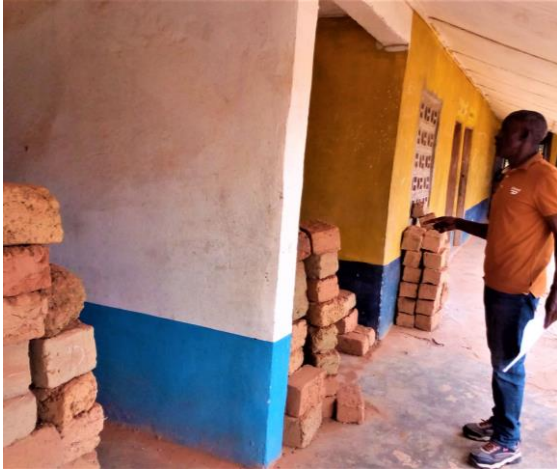
The Zwedru UMS PTA chairperson showed me mudbricks that the school made to begin the fence project. February 18, 2022.
