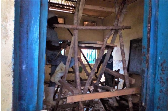
Renovation work at Harrison Grigsby UMS in preparation for the opening of school, October 19, 2021.
