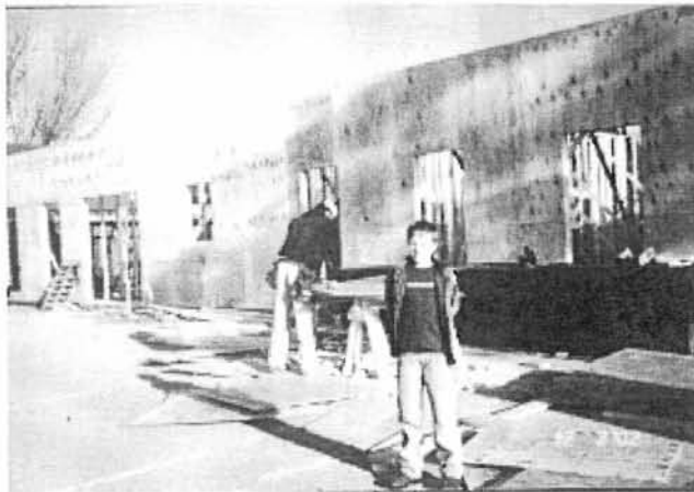
Blake White visits the work site of the new addition in December 2002.
