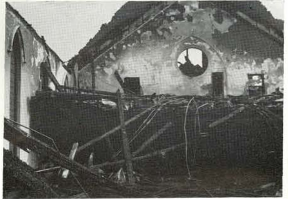
The rubble inside the burned-out church.
