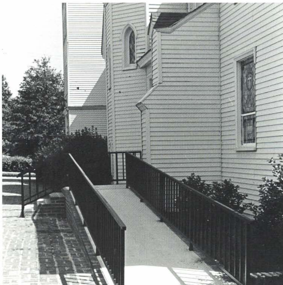
The outdoor ramp was added to the church in 1982, as a memorial to John Howard Myrick by his wife and family.
