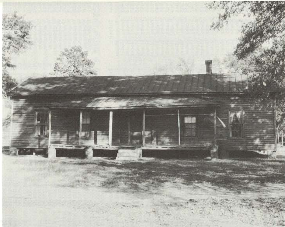
The famed old Bethel Academy, where many old Methodists were educated. It is in a bad state of repair.
