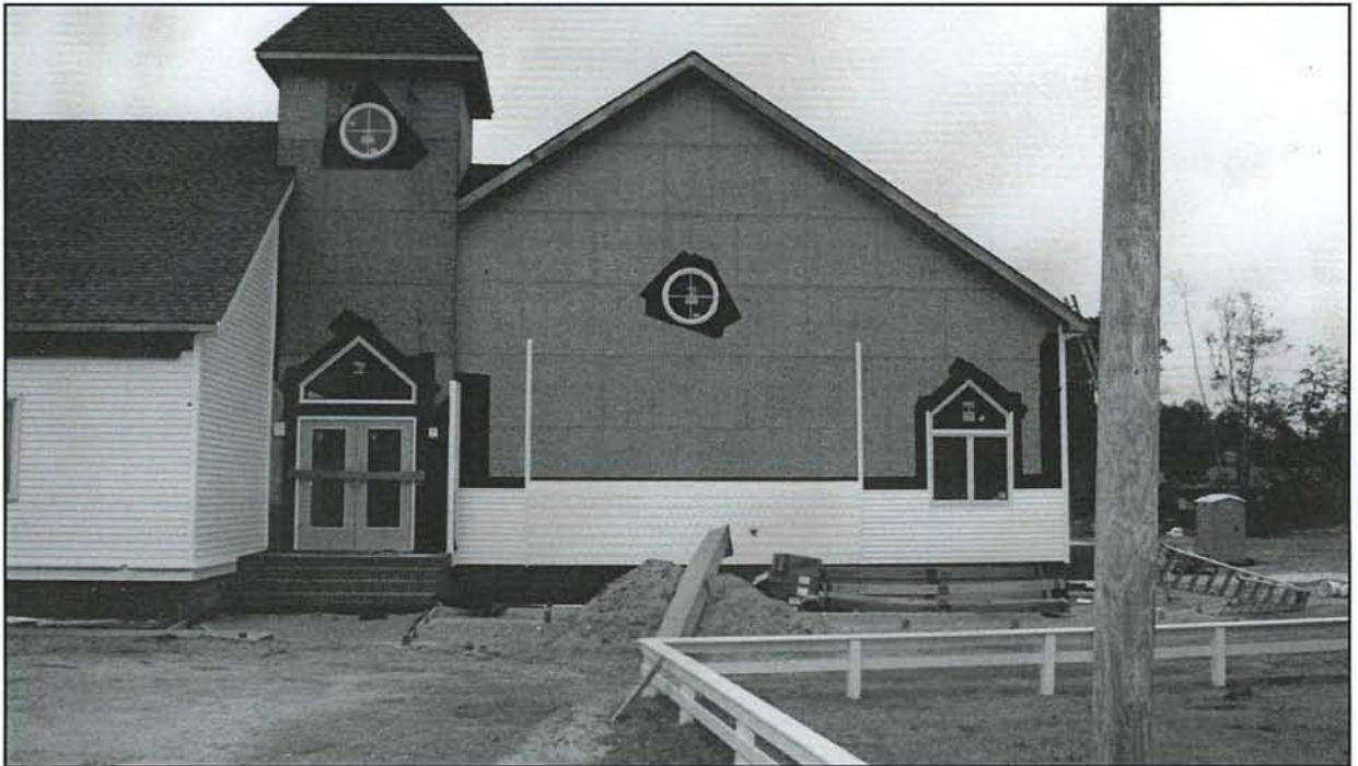
DECEMBER 2004 found the outer building mostly completed, but much to do on the inside. (Minta Meekins photo.)
