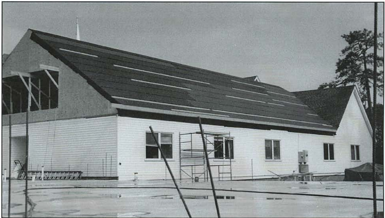
AFTER: The first stage of the building project in July 2004 was to put an A-line roof over the 1975 education addition. The unfinished attic is a large and spacious place. (Minta Meekins photo.)
