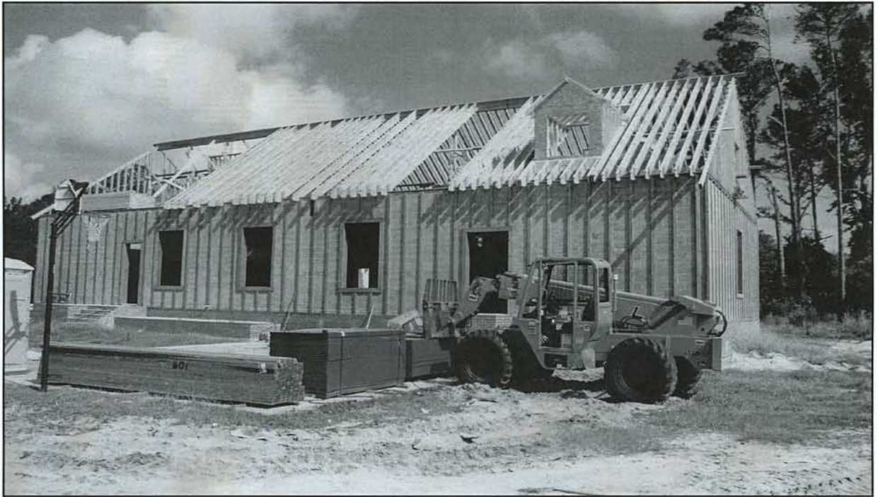
THE KITCHEN AND FELLOWSHIP HALL phase of the project is well underway in September 2004. (Minta Meekins photo.)
